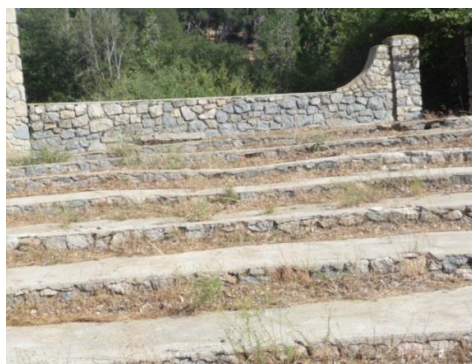
The stadium steps in disrepair
